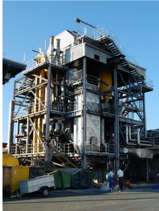
Figure 12 Güssing facility in Austria.
